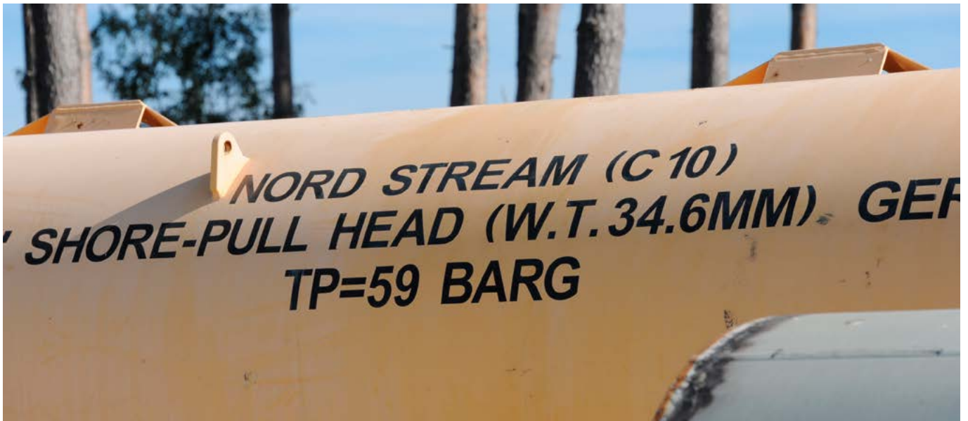
Nord Stream 1 pipeline in Lubmin, Germany. shutterstock.com / nitpicker
